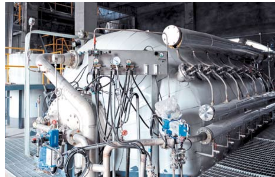
▲ LimeWhite™ for white liquor filtration in the white liquor plant.
