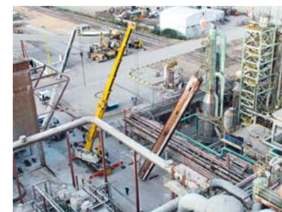
▲ The recovery boiler at Setúbal was recently rebuilt. This was a large retrofit project. Each economizer section (shown here being removed from the boiler) was 25 m high and weighed 22 tonnes.
