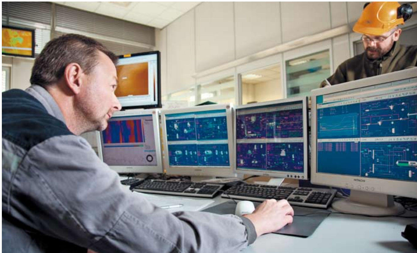
▲ One of the kiln operators oversees operations from the control room. The BrainWave® layer of KilnACE® is utilized 100% of the time.
