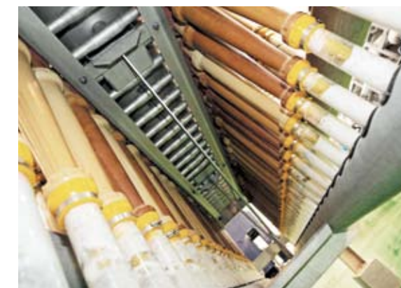
▲ ANDRITZ installed a second cleaning line to help Yueyang meet its high targets for dirt speck removal.
