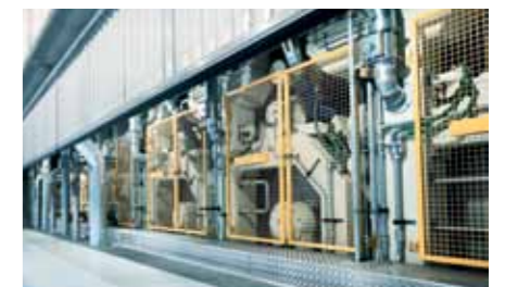
▲ View of the pre-dryer section with vacuum rolls and web stabilizers.
