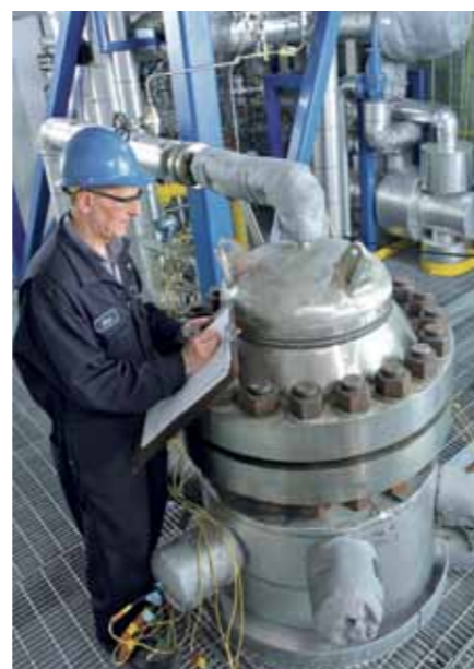
▲ Richard Knight, GTI Project Manager, shown with a portion of the TIGAS equipment at the Flex Fuel facility.
