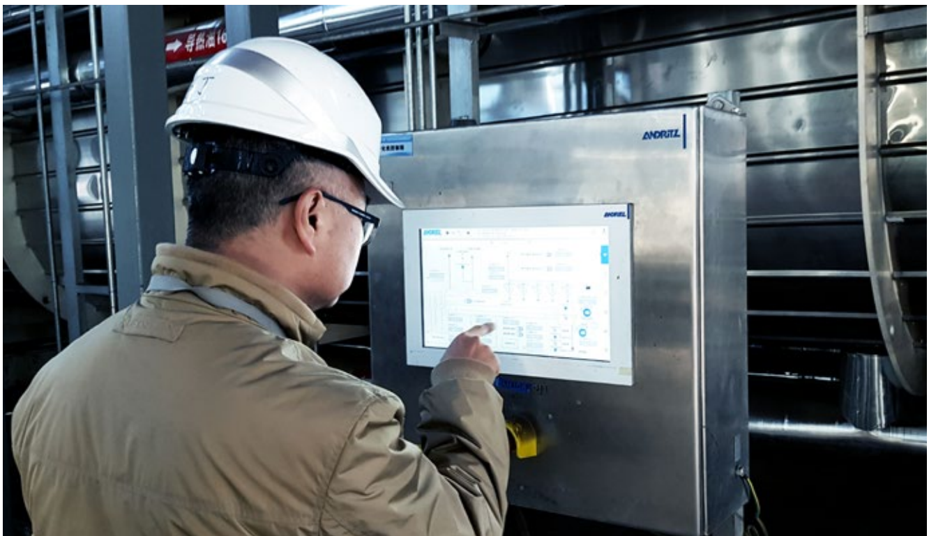
Automated operation systems
